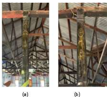
Fig. 10. Old Church Pillar Asei (a) Left side of Hawa and (b) Right side of Adam
