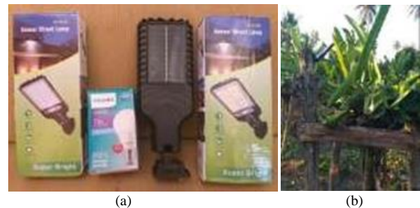
Fig. 8. Installation of solar cell lights in the Dragon Fruit Garden area: (a) Cell Solar Lamp; (b) Installation of lights
