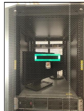
Fig. 5. System developed and installed.
