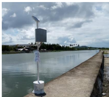
Figure 8. The System Installed Alongside the Surigao River
