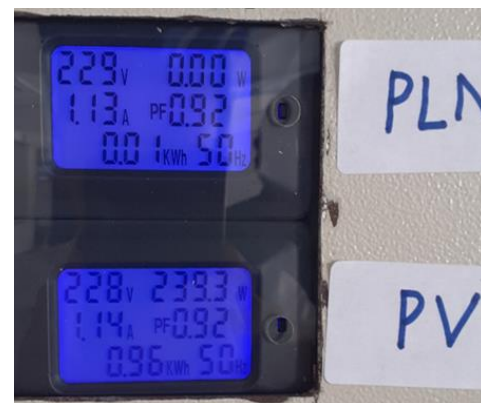
Fig. 3. The output of PLN and solar panel
