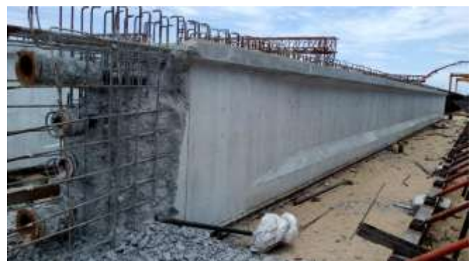
Fig. 1. View of the PSC Girders of Pipe Conveyor Bridge of 2 X 660 MW Udangudi Super Critical Thermal Power Project at Thiruchendur
